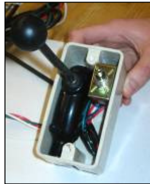
Figure 16. Photo of toggle switch (right) before modifications were made.
