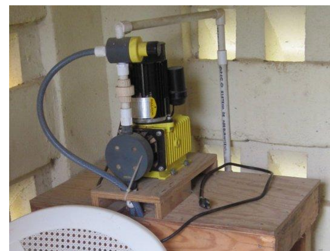
Figure 4: A new chlorinator found at a nearby village.
