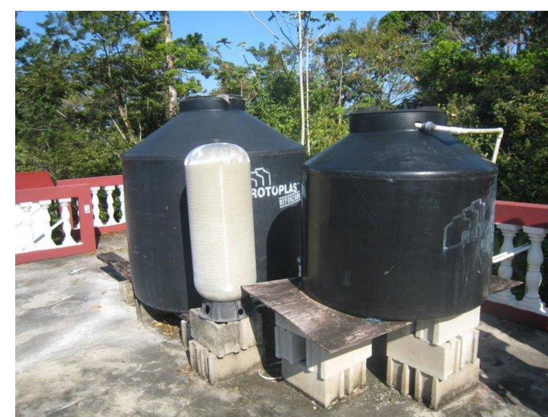
Figure 2: Water storage tanks on-top of the Hillside Clinic used for sanitation purposes.
