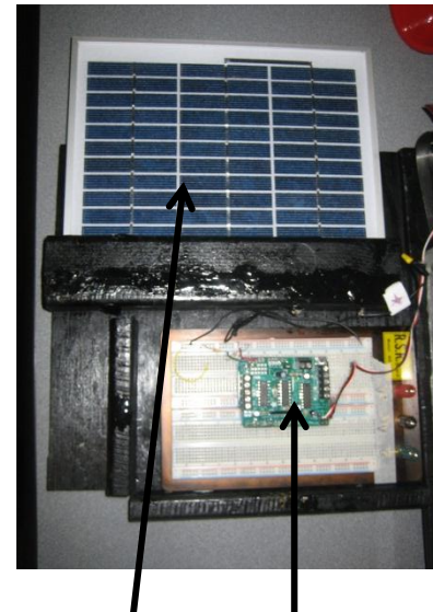
Figure 6: Solar panel and microcontroller of the BrightWater system.
