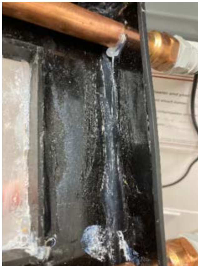
FIGURE 1: Caulk Lining (DRIED)
