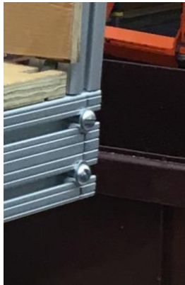
Figure 21 : Bolts used to fasten the frame together after internal fastener failure.
