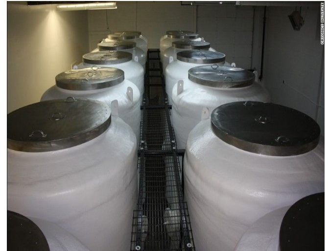
Figure 2: Large capacity LN2 storage tanks at the University Hospitals Cleveland Medical Center.
